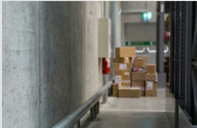
Blocked emergency exit detection
